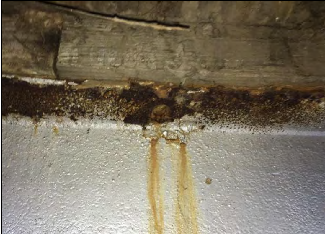
Photograph 14: Missing bolted connection and corroded top flange of bridge girder in Bay F.
