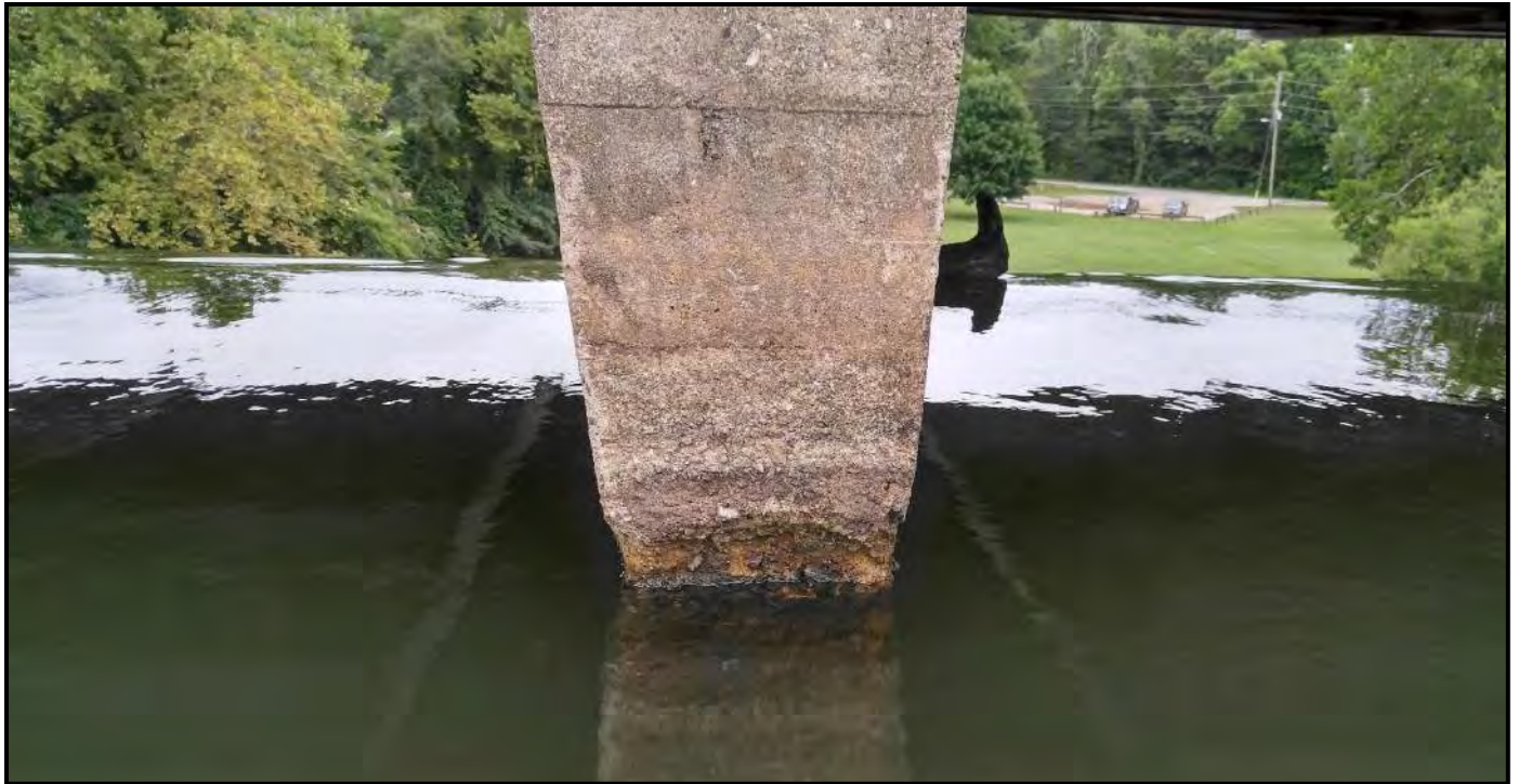
Photograph 37: Wearing of the concrete bridge abutment at the water level.
