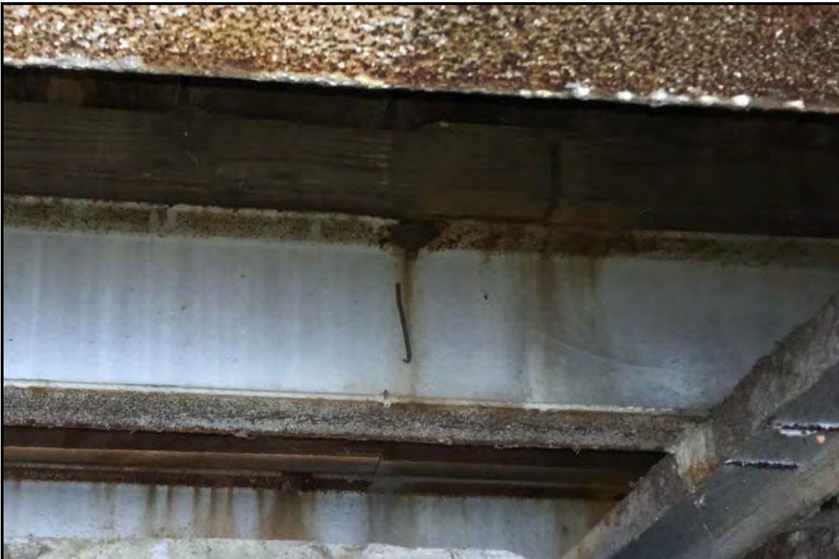
Photograph 12: Severely corroded bolted connection and top flange of bridge girder in Bay K.
