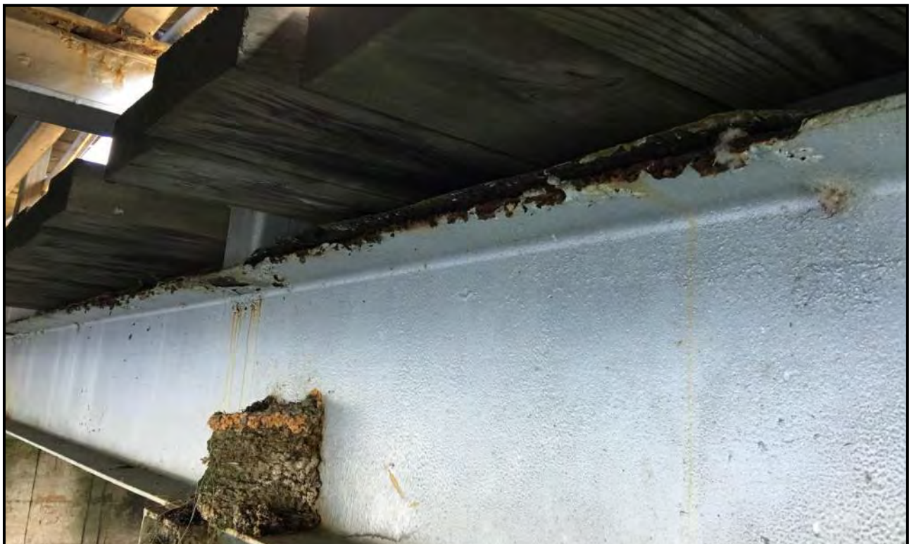
Photograph 26: Severe corrosion and delamination of top flange of bridge girder/post support beam in Bay C.
