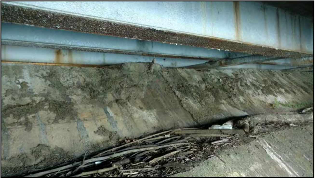
Photograph 1: Missing intermediate concrete abutment for 8" bridge girder support at Bay M.
