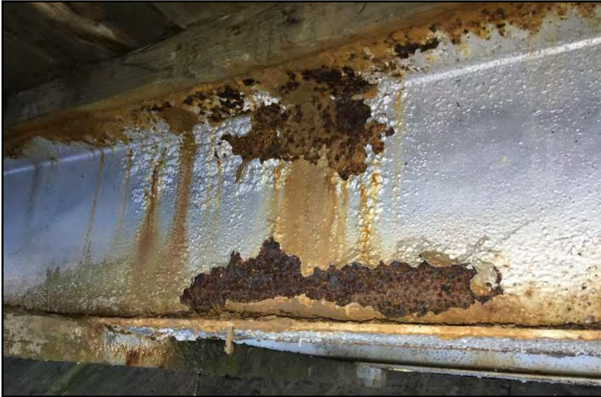
Photograph 17: Corrosion of bolted connection, top flange, and web of bridge girder in Bay B.
