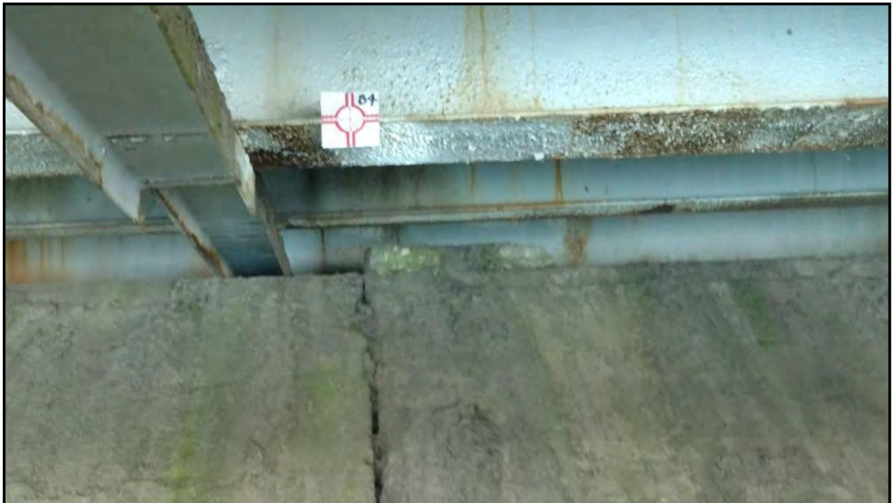
Photograph 6: Damaged intermediate concrete abutment for 8" bridge girder support at Bay B.
