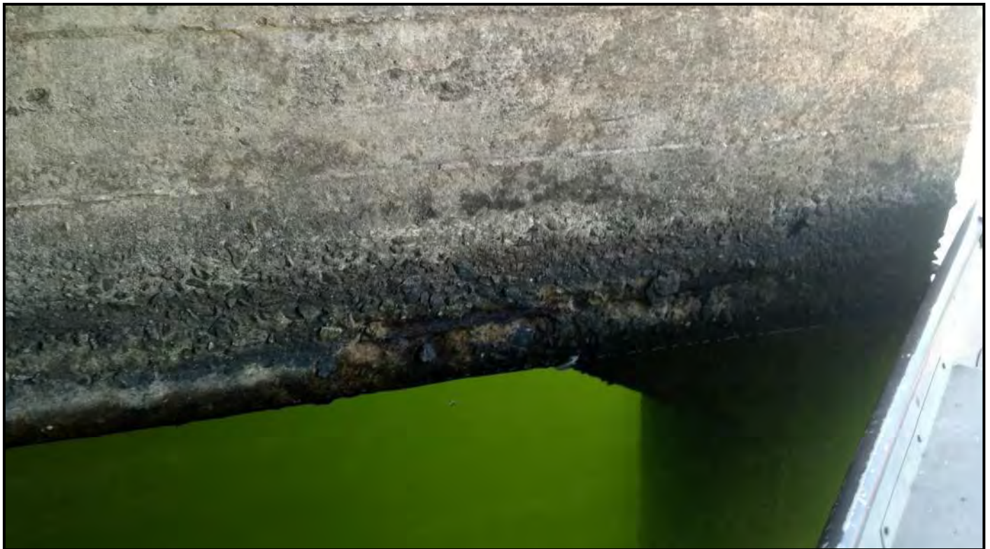
Photograph 38: Wearing of the concrete bridge abutment at the water level.
