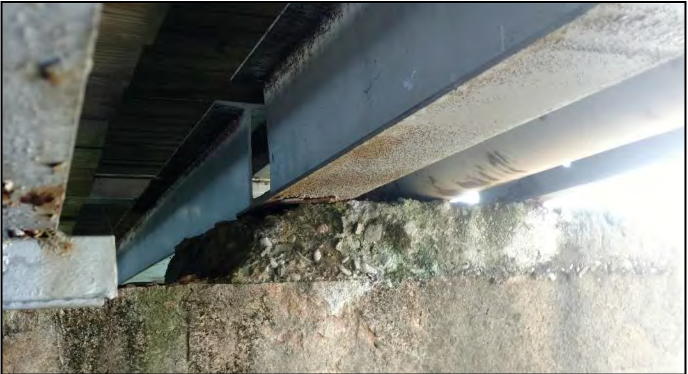
Photograph 33: Damage to built-up section of the concrete bridge abutment at bridge girder bearing location.
