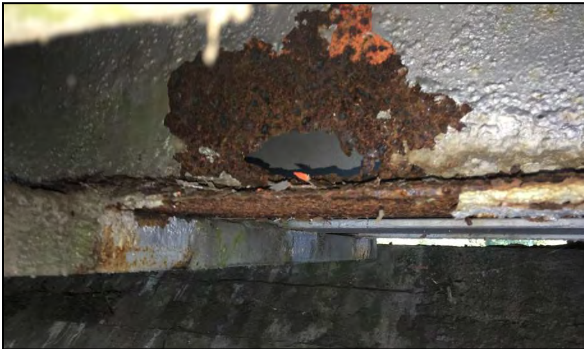
Photograph 24: Severe corrosion of web and bottom flange at mid-span of bridge girder in Bay O. Supplemental girders added on either side in early 1990's.
