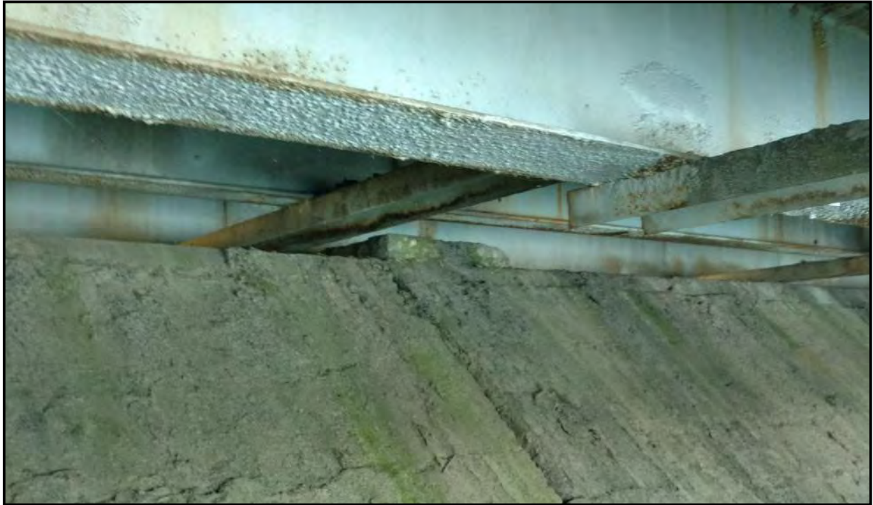
Photograph 5: Damaged intermediate concrete abutment for 8" bridge girder support at Bay B.
