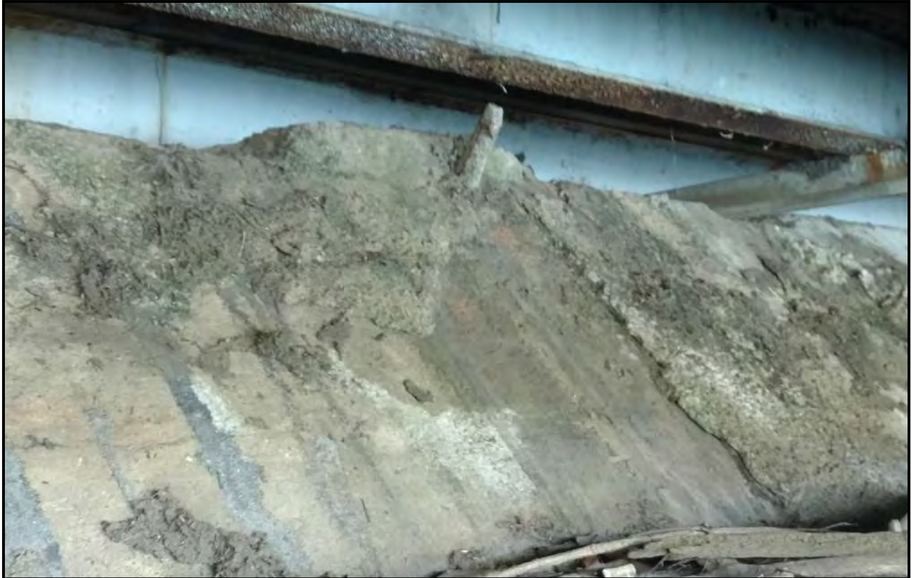
Photograph 2: Missing intermediate concrete abutment for 8" bridge girder support at Bay M.
