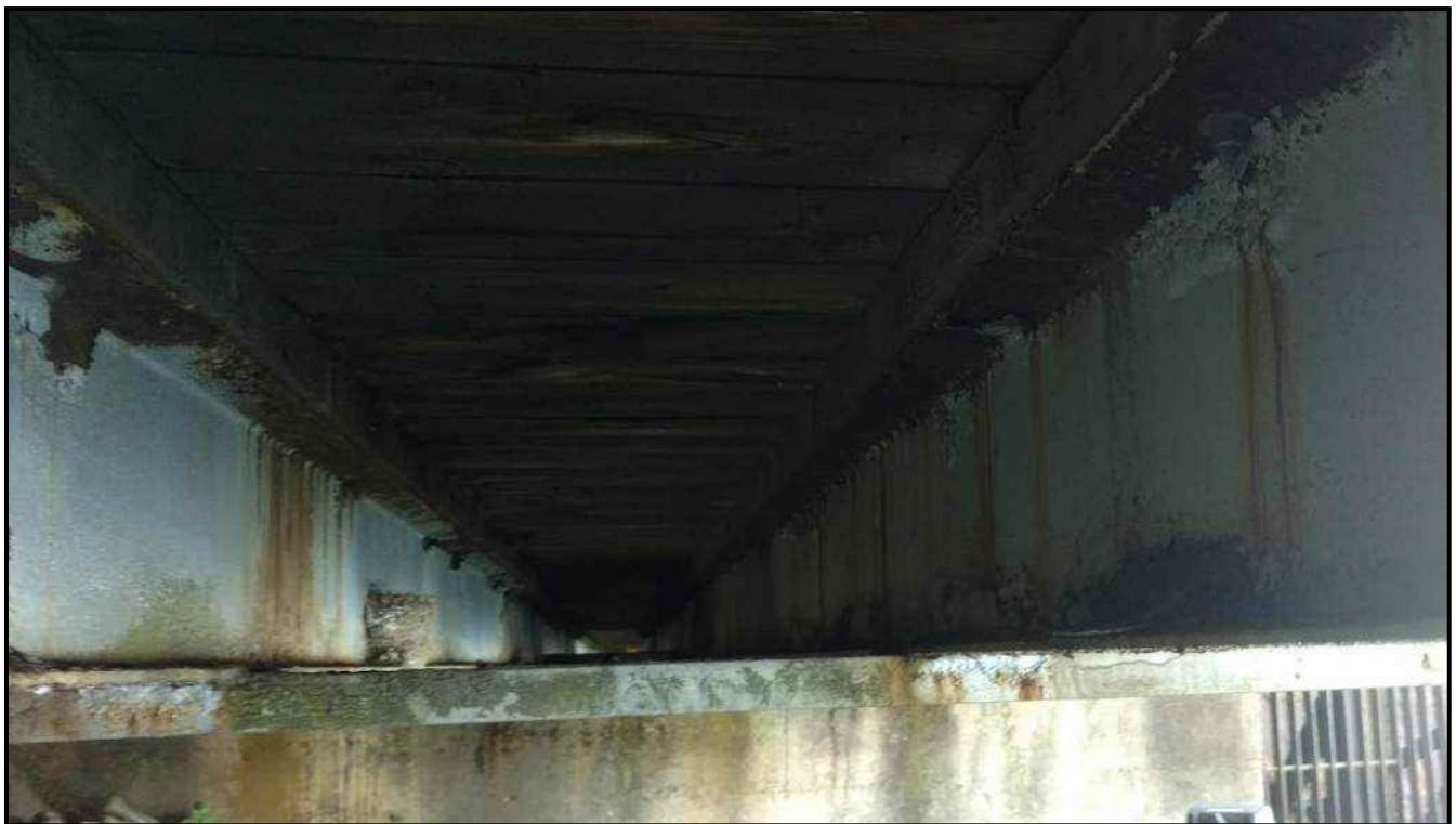
Photograph 22: Corrosion of bolted connections and top flanges of bridge girder at Bay M.
