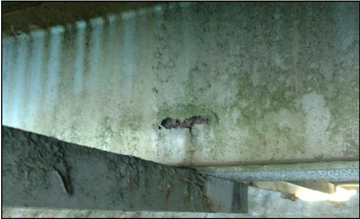
Photograph 29: Damage and corrosion at back side of weld for the lateral bracing member.
