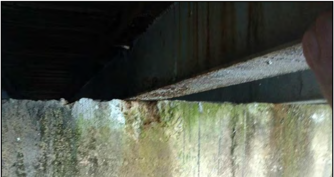
Photograph 32: Damage to concrete bridge abutment at Bay M – Bay L bridge girder bearing location.
