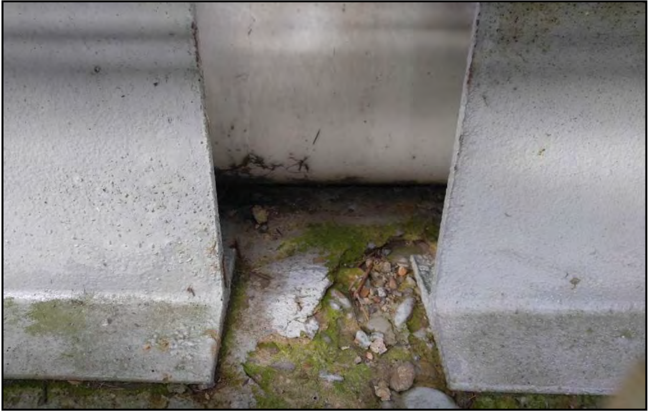
Photograph 31: No bearing plates at bridge girder bearing locations.
