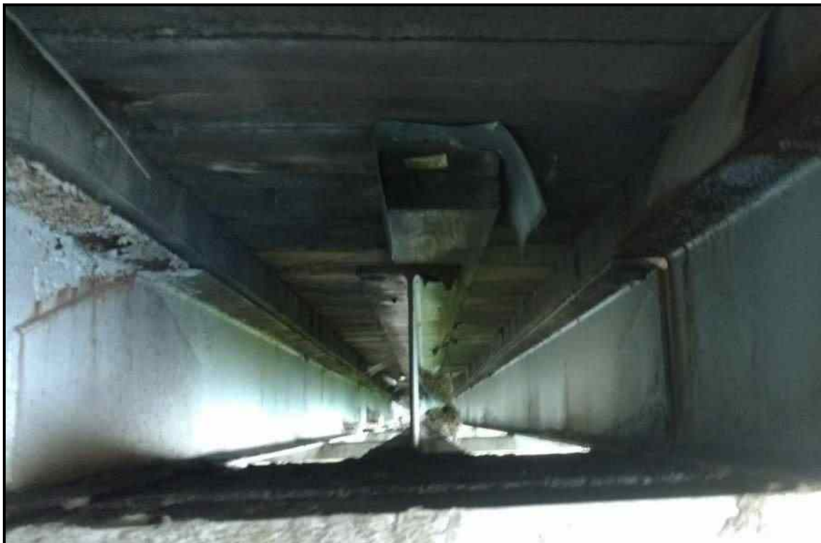
Photograph 8: Insufficient connection of supplemental bridge girder to bridge deck.
