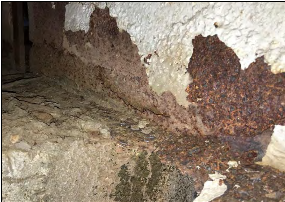
Photograph 20: Severe corrosion of web and bottom flange of bridge girder at Bay K – Bay L bearing location.
