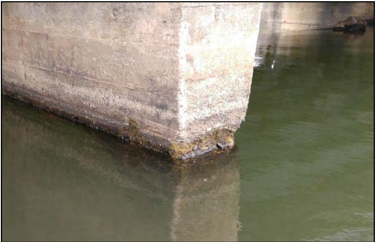
Photograph 36: Wearing of the concrete bridge abutment at the water level.
