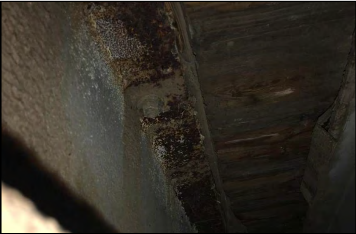
Photograph 11: Severely corroded bolted connection and top flange of bridge girder in Bay Q.
