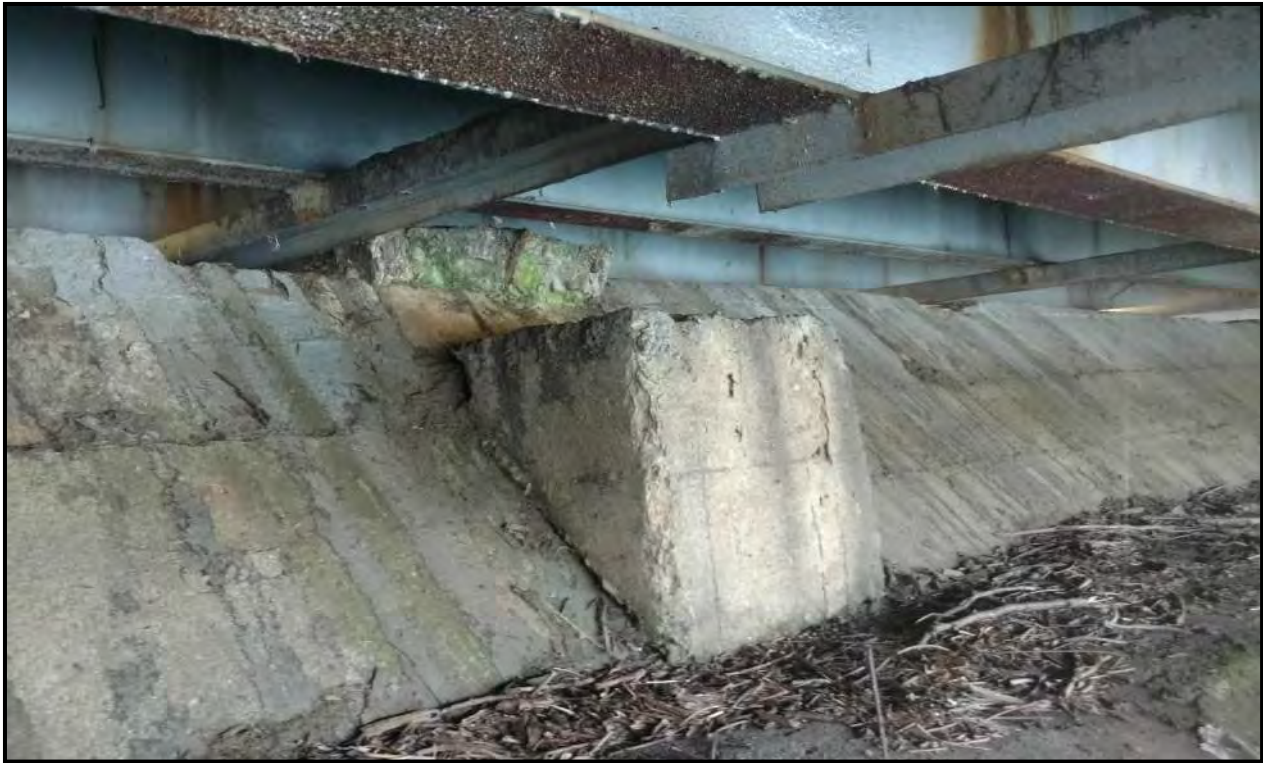
Photograph 3: Damaged intermediate concrete abutment for 8" bridge girder support at Bay K.
