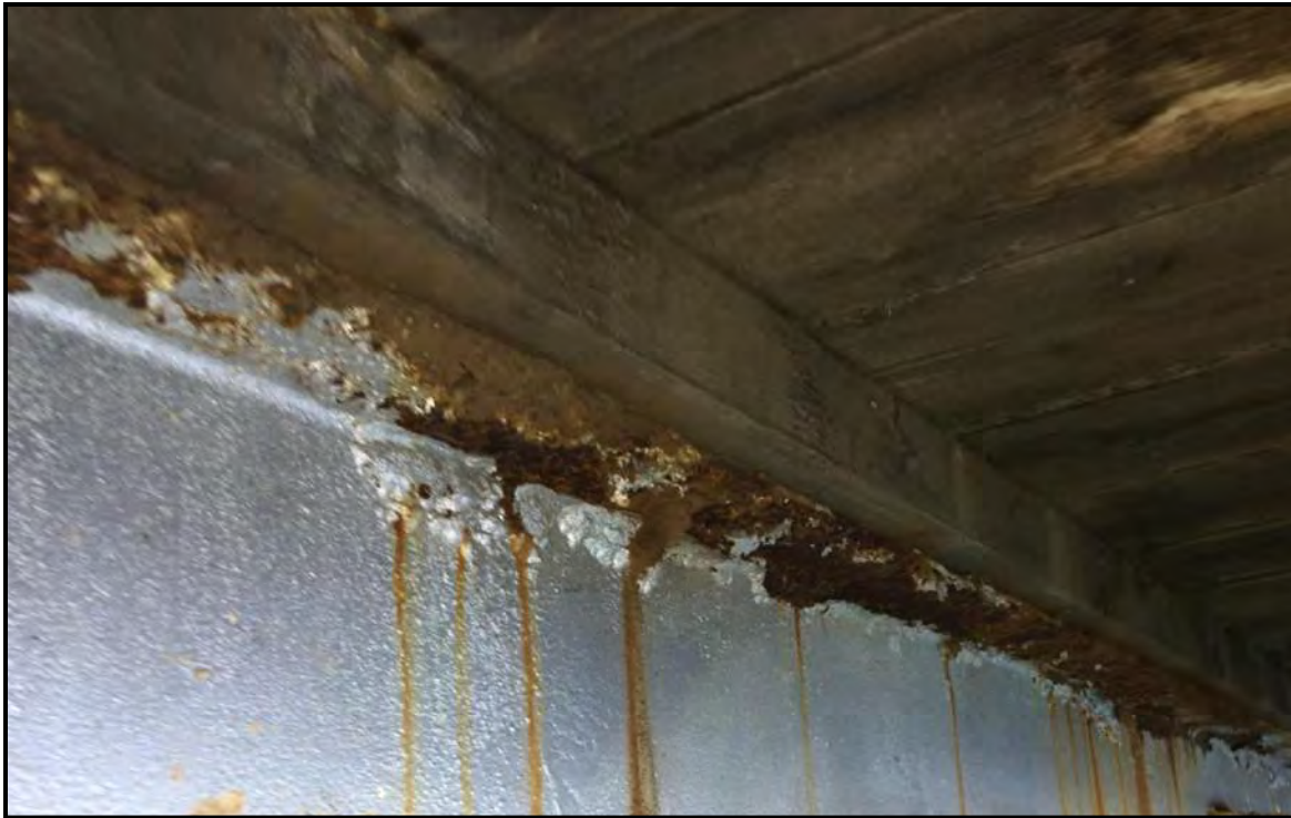
Photograph 13: Severely corroded bolted connection and top flange of bridge girder in Bay M.
