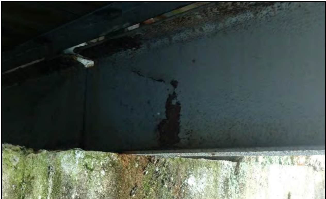
Photograph 28: Damage and corrosion at back side of weld for bridge girder connection plate typical at bridge girder connection plates.
