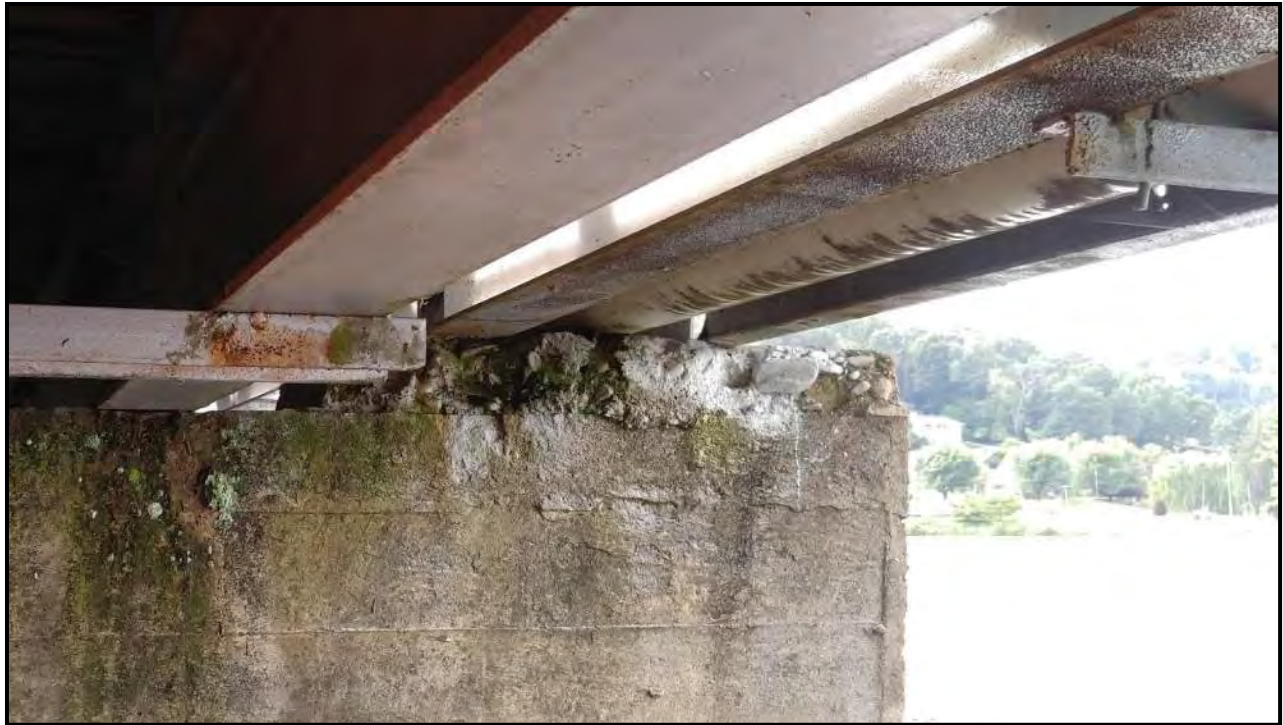
Photograph 35: Damage to built-up section of the concrete bridge abutment at bridge girder bearing location.
