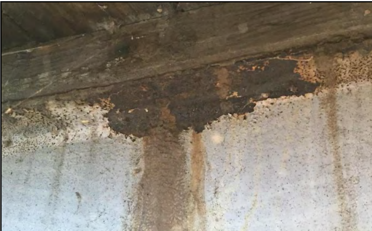
Photograph 18: Missing bolted connection and corrosion of top flange of bridge girder in Bay D.
