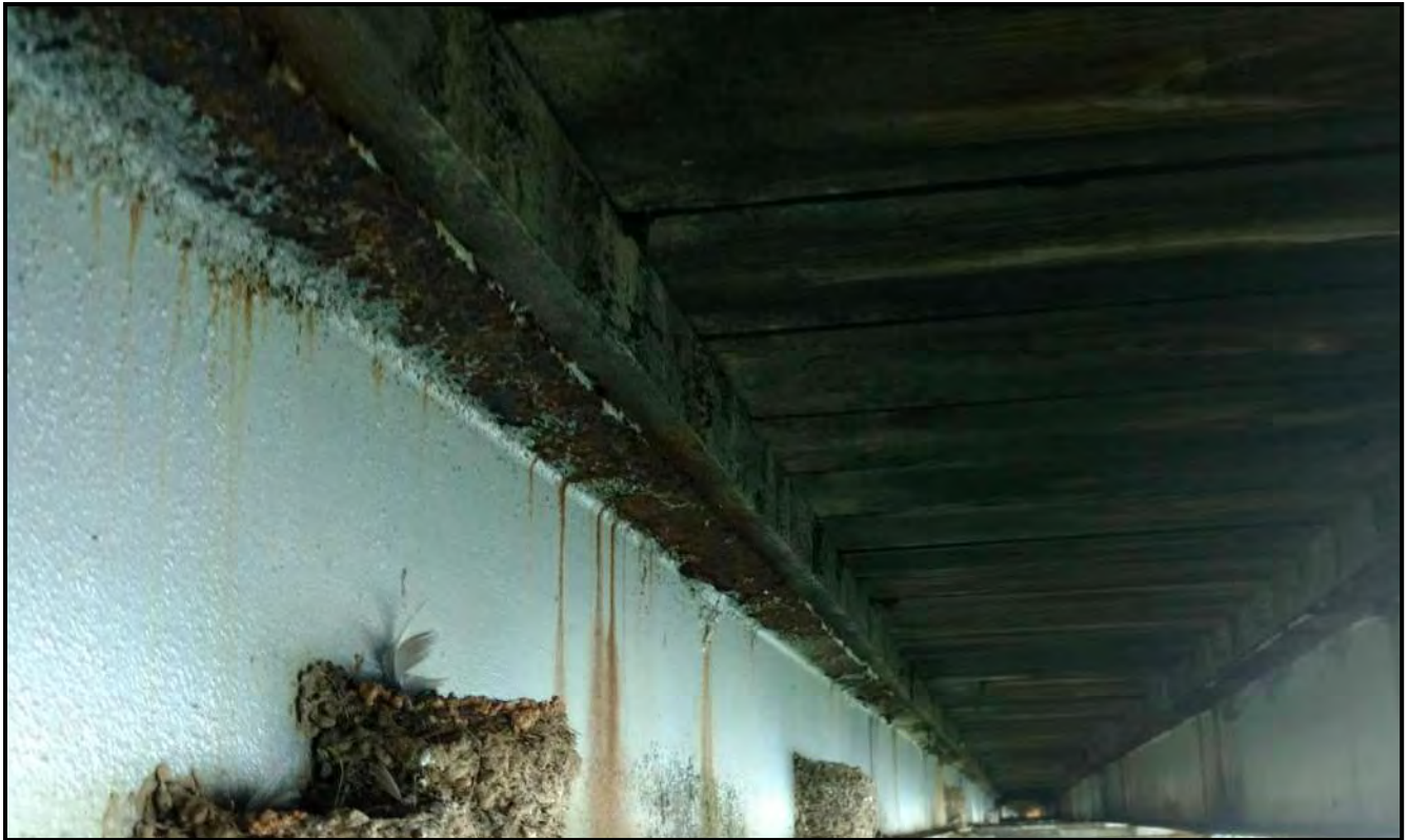
Photograph 21: Corrosion of top flange of bridge girder at Bay N.
