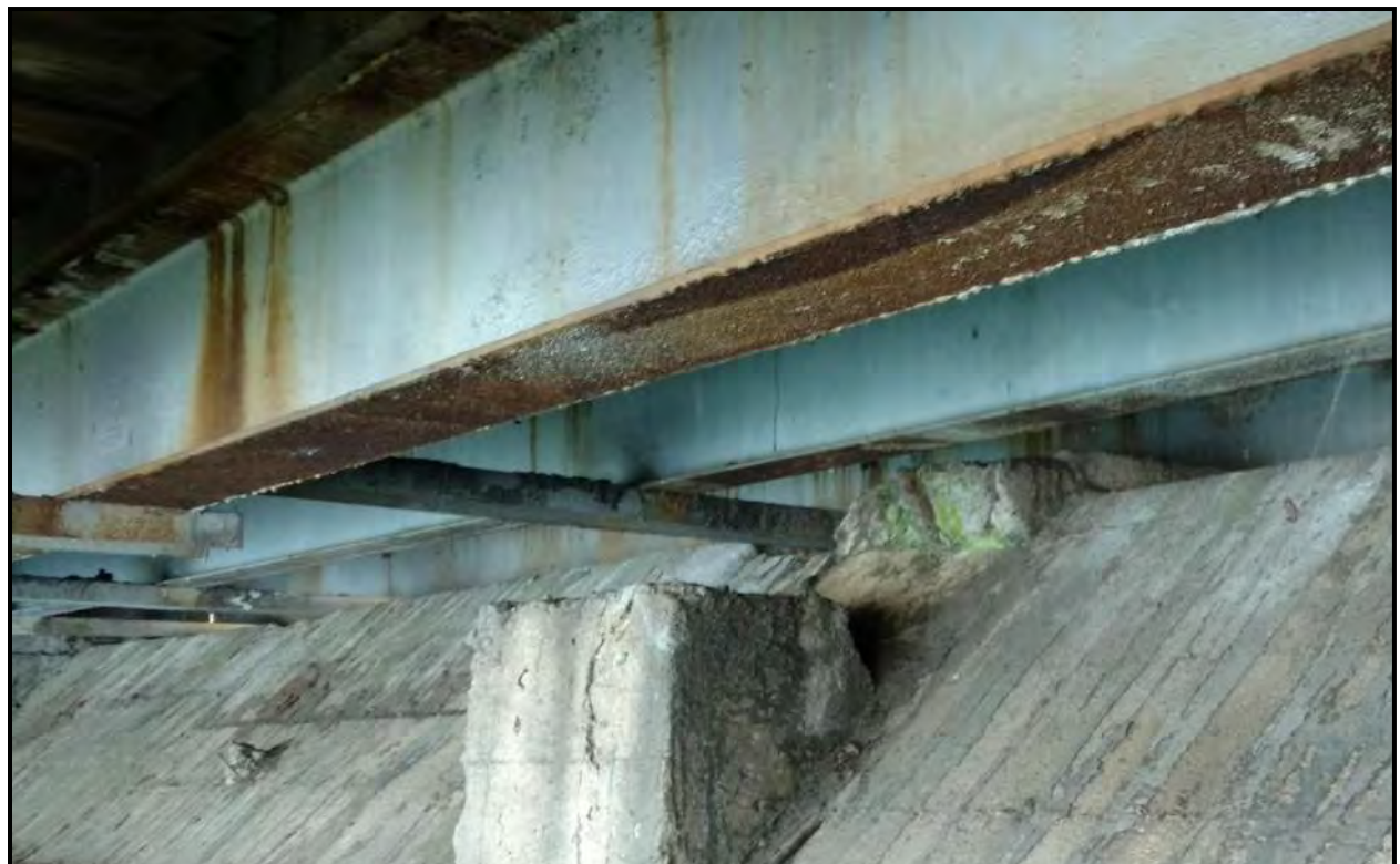
Photograph 4: Damaged intermediate concrete abutment for 8" bridge girder support at Bay K.
