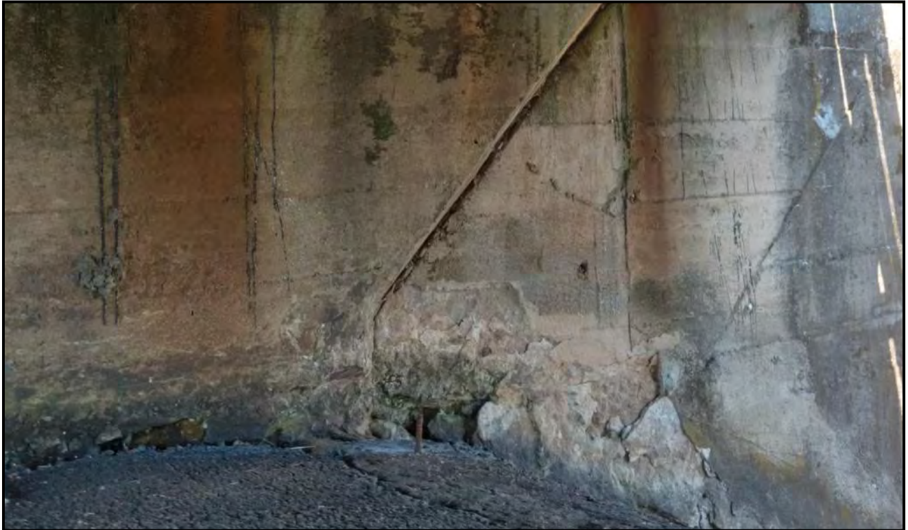
Photograph 39: Damage and spalling to the concrete bridge abutment between Bay J and Bay K at the interface with the spillway surface.
