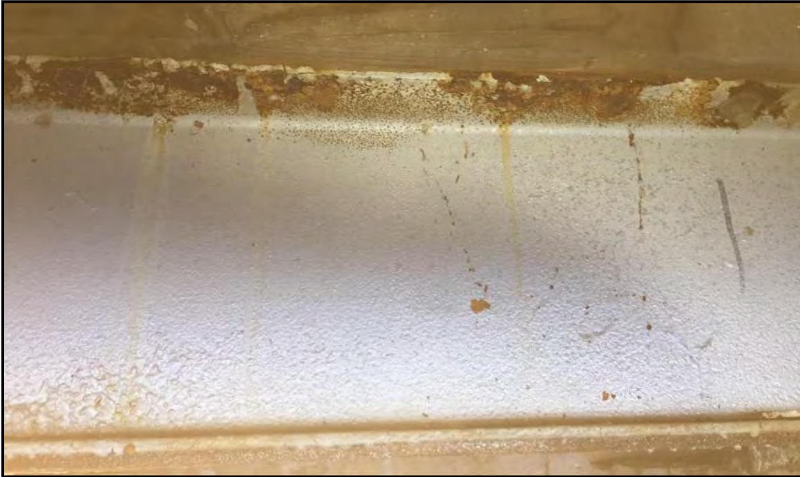
Photograph 19: Corrosion of bolted connection and top flange of bridge girder in Bay K.
