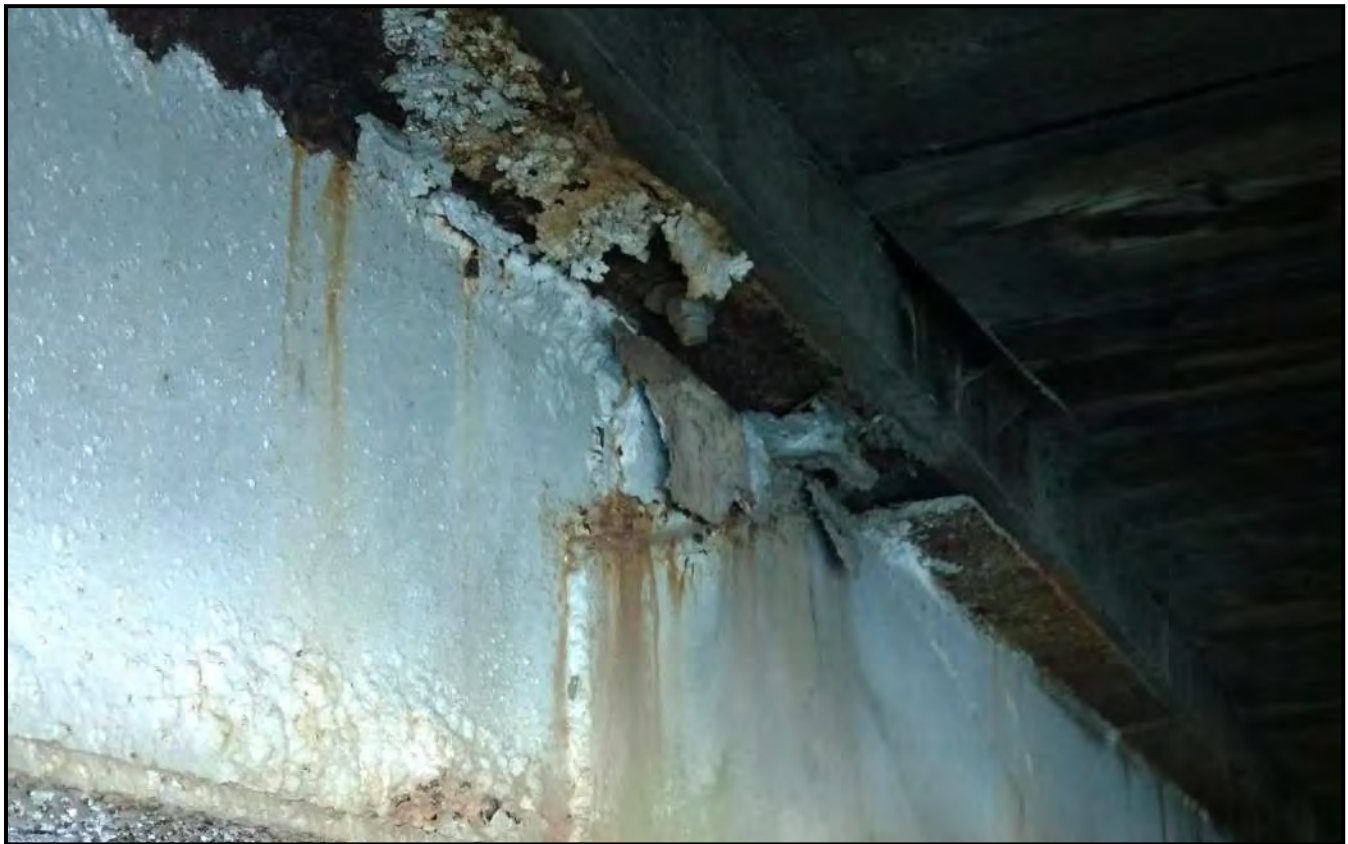
Photograph 10: Severely corroded bolted connection and top flange of bridge girder in Bay M.
