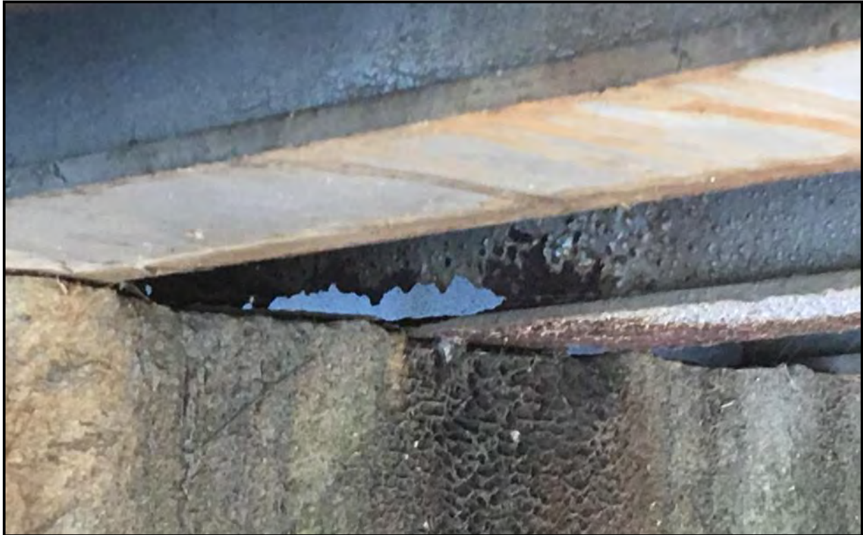
Photograph 23: Severe corrosion of web of bridge girder at Bay G-Bay H bearing. Supplemental girders added on either side in early 1990's. Supplemental girder shown in foreground.
