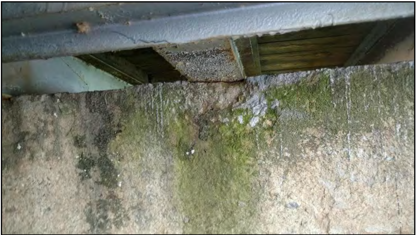
Photograph 34: Damage to the concrete bridge abutment at bridge girder bearing location.
