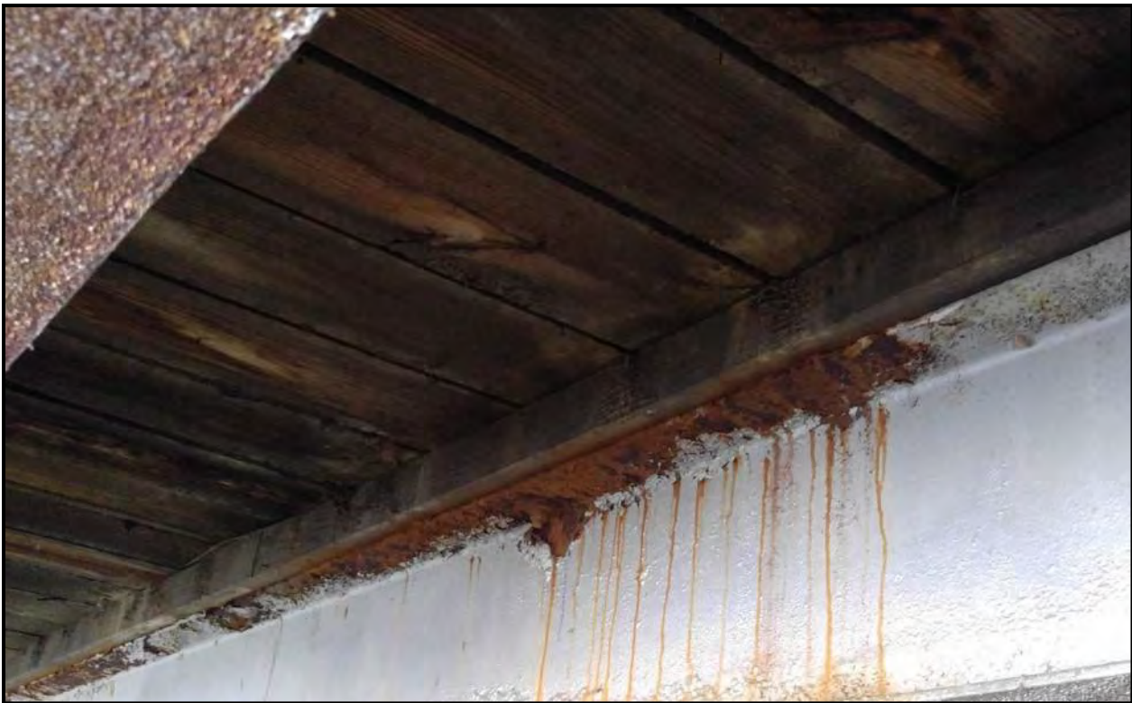
Photograph 16: Missing/Corroded bolted connection and corroded top flange of bridge girder.
