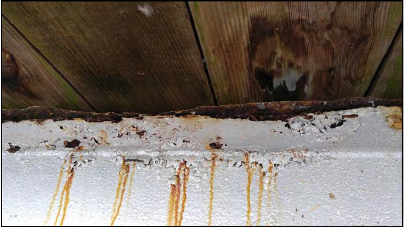
Photograph 27: Severe corrosion and delamination of top flange of bridge girder/post support beam in Bay M.
