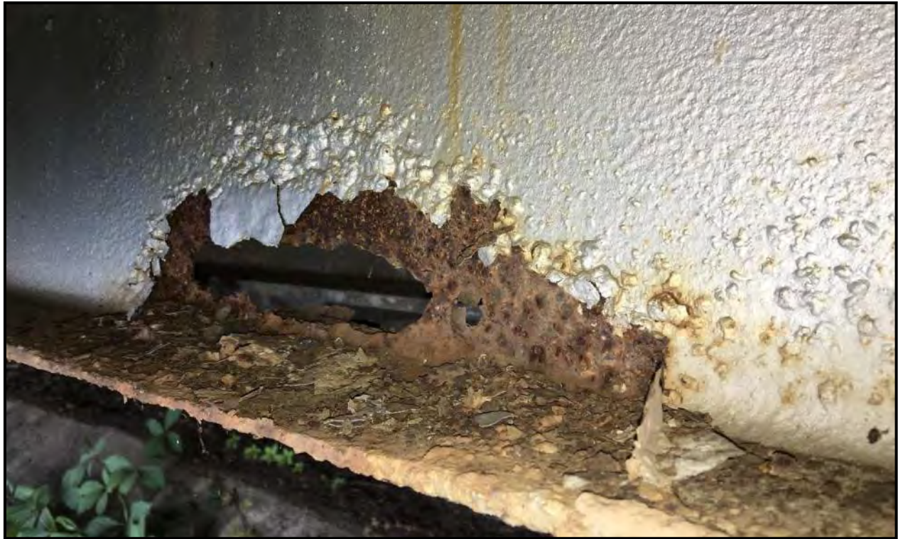
Photograph 25: Severe corrosion of web and bottom flange at mid-span of bridge girder in Bay Q. Supplemental girders added on either side in early 1990's.
