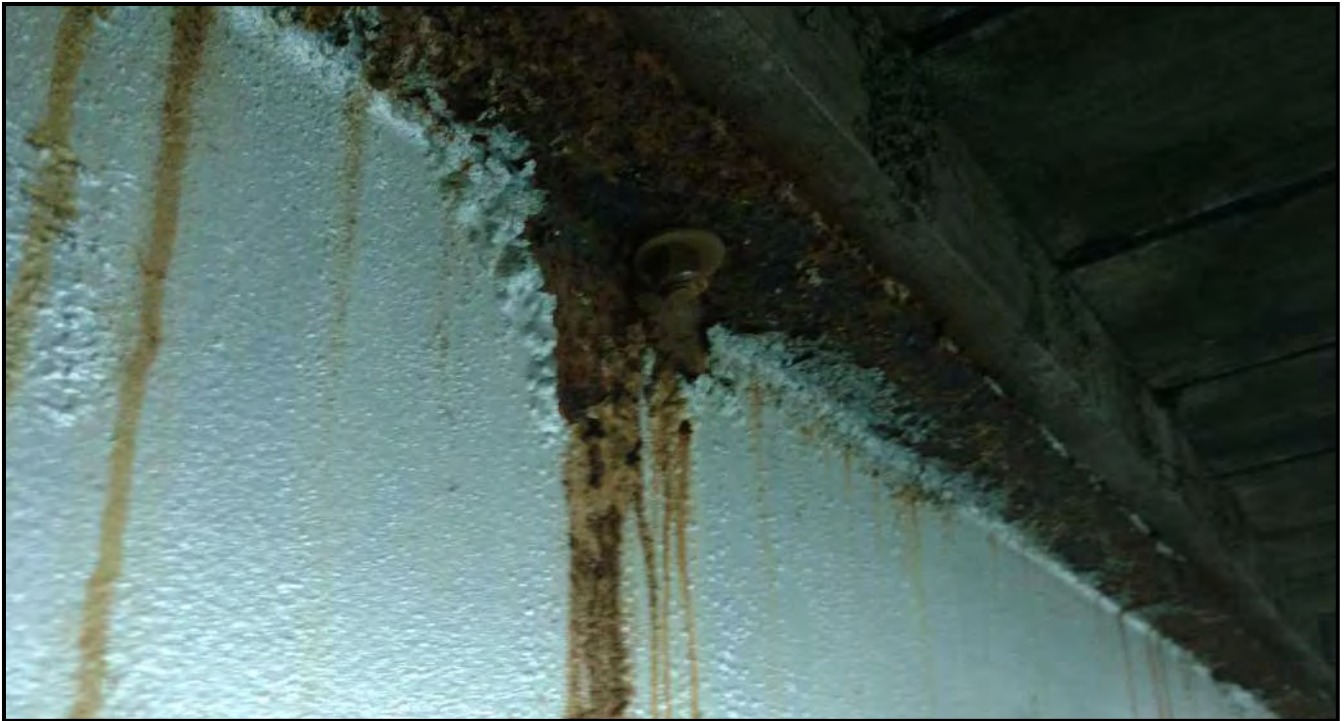
Photograph 9: Severely corroded bolted connection and top flange of bridge girder in Bay N.
