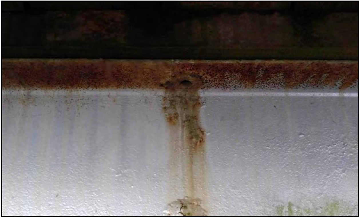
Photograph 15: Missing bolted connection and corroded top flange of bridge girder.
