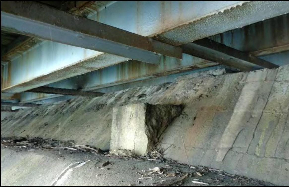
Photograph 7: Damaged intermediate concrete abutment for 8' bridge girder support at Bay A.
